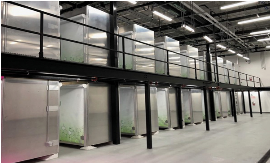
Facility with AVFUs
